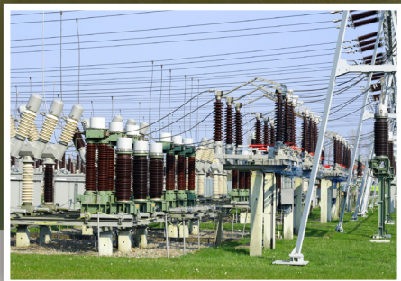
Advantech Implements Smart Wireless Routers for Substation Communication P.14
